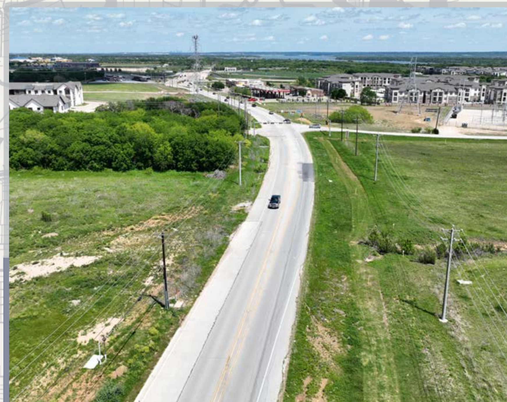
Debbie Lane construction will improve mobility and the continuity of the corridor
